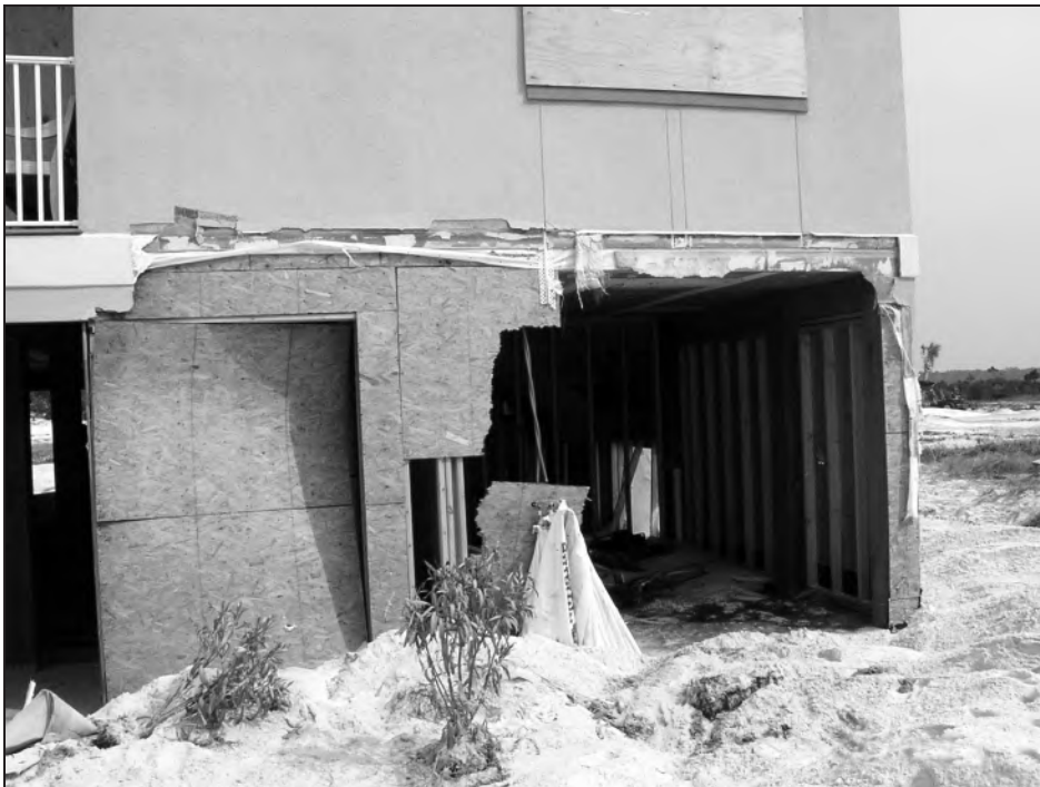
Figure 8. Non-compliant breakaway wall spanning across a vertical foundation element
