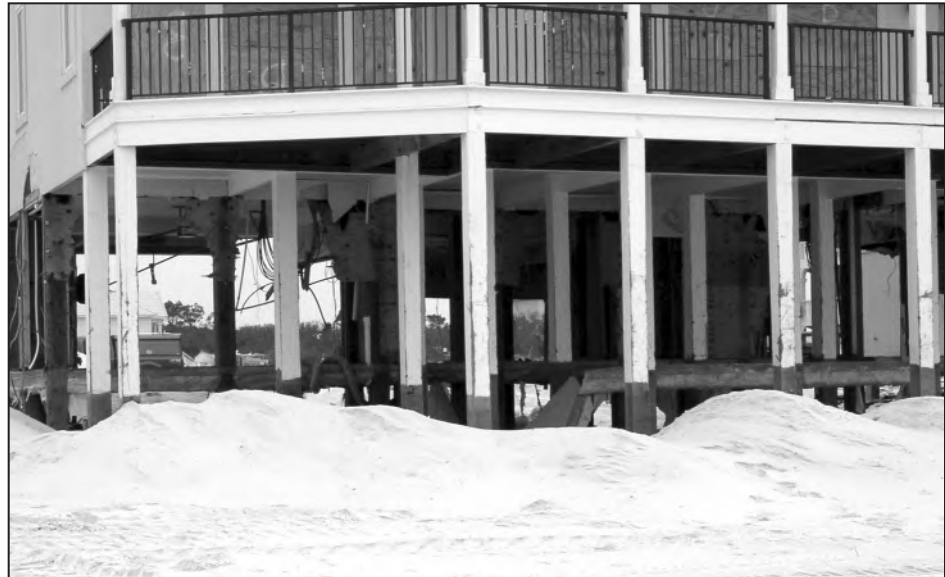
Figure 3. Successful breakaway wall performance
