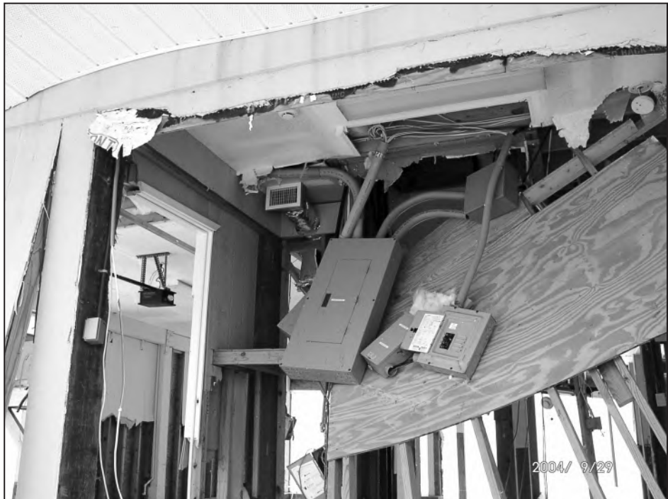
Figure 6. Non-compliant utilities attached to breakaway wall
