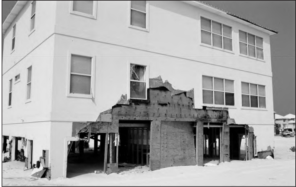
Figure 5. Non-compliant breakaway wall joint detailing
