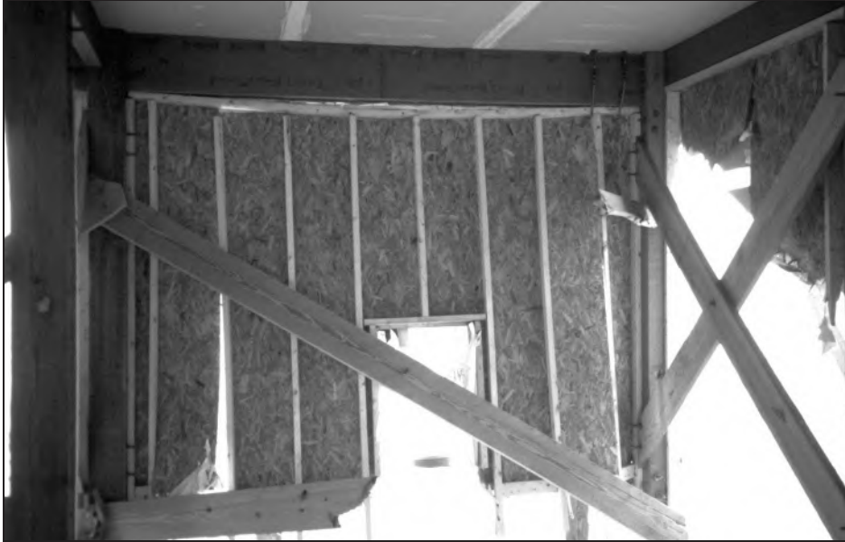
Figure 7. Non-compliant bracing arrangement
